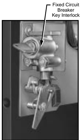
SEF Circuit Breaker with Key Interlock
